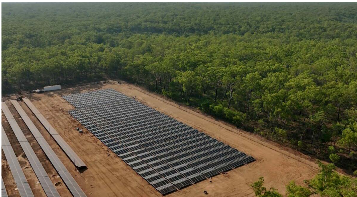
Aerial view of the Wurrumiyanga Solar Infill and Energy Storage Pilot Project. Photo: 5B.
